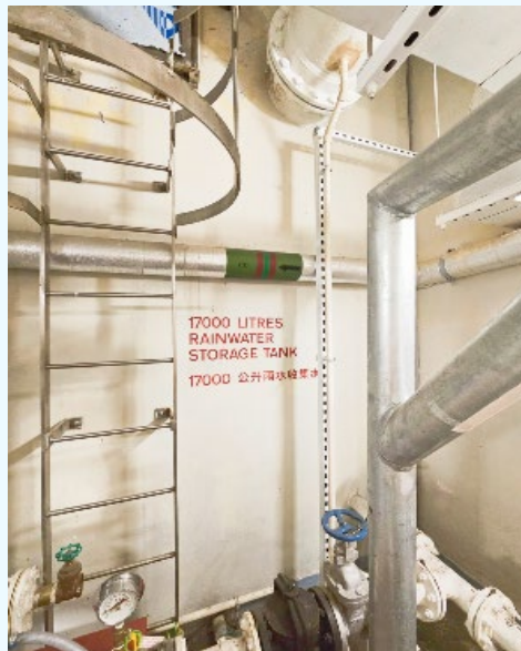
Figure 5-13: Rainwater storage tank
