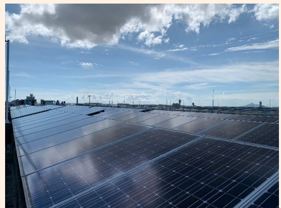
Figure 5-5: Photovoltaic panels installed at rooftop
