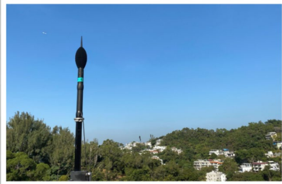
Figure 2-4: Outdoor noise monitoring terminal
