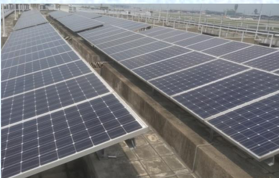
Figure 5-5: Photovoltaic panels on the rooftop of CAD Headquarters
