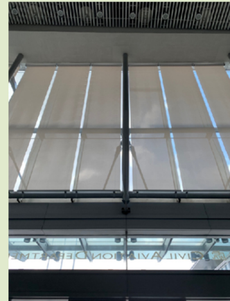
Figure 5-5: Motorized blinds at the atrium of CAD Headquarters shield sunlight effectively
