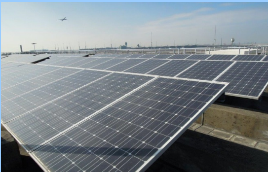
Figure 5-6: Photovoltaic panels on the rooftop of CAD Headquarters
